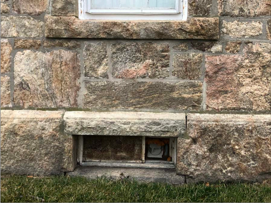
Photo 35. Original ventilator windows fitted within the foundation walls and servicing the cellar played a large role in the health and stability of the Lighthouse and its occupants: Disallowing the buildup of radon, illuminating and ventilating the cellar and – via convection – upper occupied floors, oxygenating the original lamp, and optimizing ambient moisture. Blocked, they provide no benefit and allow for the ingress of water to occur unnoticed.
