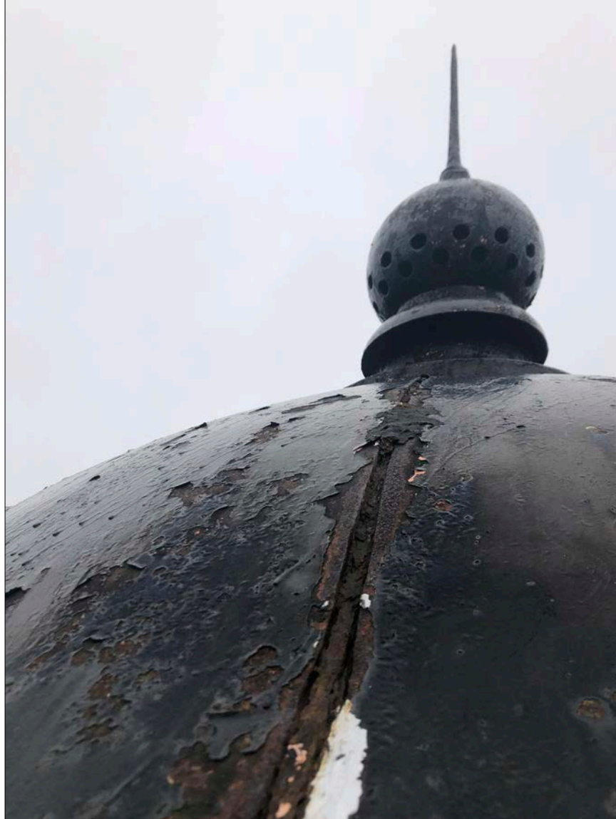
Photo 14. View of six-panel ogee dome atop Lantern, including ventilator ball. The original terminal is not connected to a lightning protection system. Open joints are severe and allow water to migrate into Lantern (leading to the funnel & tube collection apparatus at the interior cove); joints, surfaces and features of this roof are all imminently restorable.
