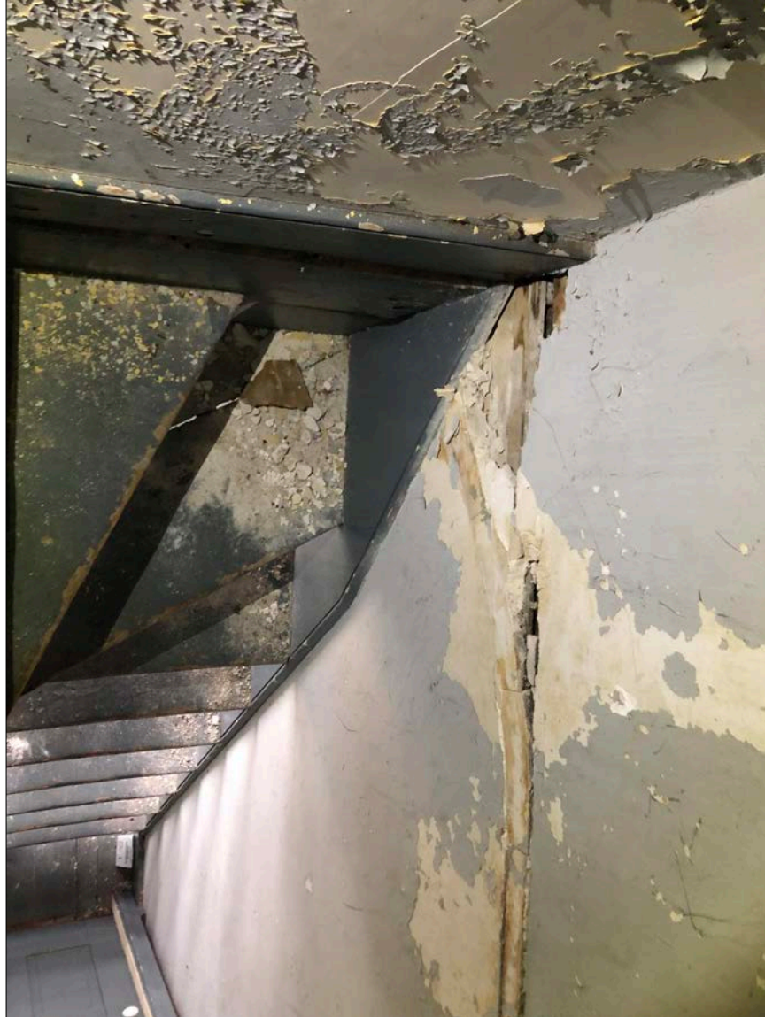
Photo 49. Generally, interior surfaces suffer from migration of stormwater – which has corrupted and deteriorated the original plaster wall finishes and other systems – and a lack of regular cleaning of those interior spaces that are only intermittently used.
