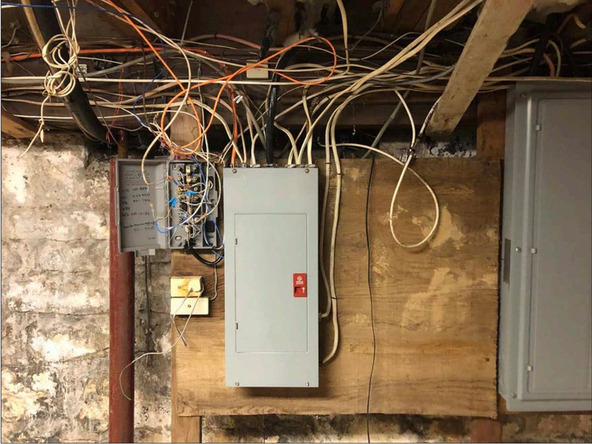
Photo 47. Electrical service is a series of ad hoc modifications, lacking an overarching benchmark of quality control. Beneath this panel is precisely where regular flooding forms, just inside the base of the southeast bulkhead entrance. Flooding is caused by an inadequate stormwater collection & distribution system.
