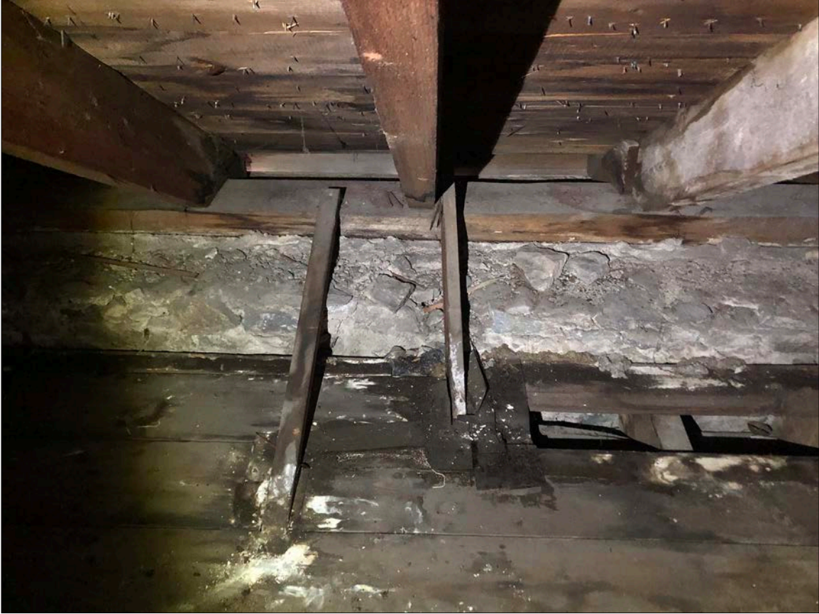
Photo 37. Ties, sister joists, and other interventions have occurred at both the roof rafter structural framing system and, illustrated below, floor plate framing. This has universally been necessitated by the inability of the roofing, flashing, gutters, downspouts and subsurface connections to properly and consistently collect and move stormwater safely away from the building. White stains on the right framing member in the image indicates water staining and residual water-borne particulates (salt).
