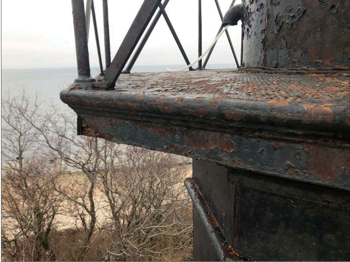
Photo 19. View of Watch Deck fascia, looking northeast. Note deep corrosion at miter on left, which corresponds to the rail anchors, and their relative watertight integrity.
