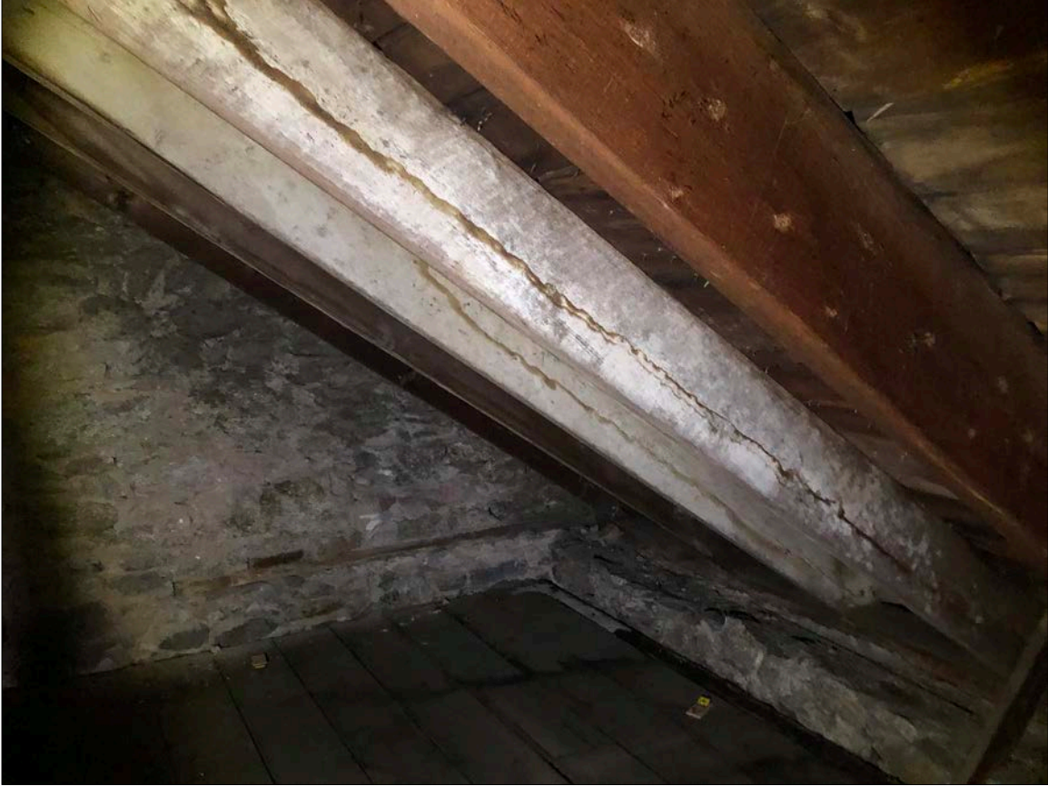
Photo 38. Another view in the attic shows the extent of prolonged water migration... and damage.
