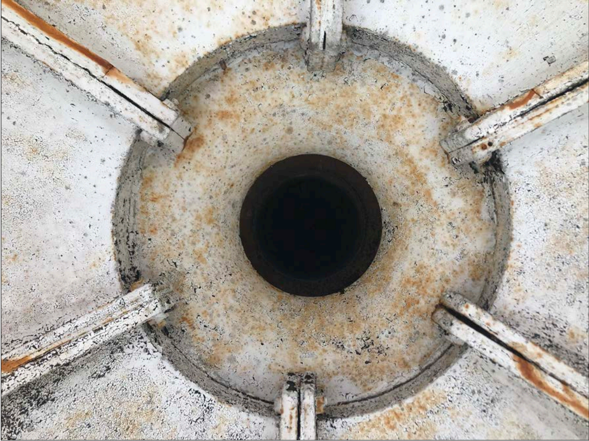
Photo 10. View to top of Lantern at culmination of the iron spider frame. The opening at center leads to the spherical vent ball mounted at the roof apex, which controls crucial convective air currents from grade to Lantern. This current continually refreshes the air at all levels of the Lighthouse.
