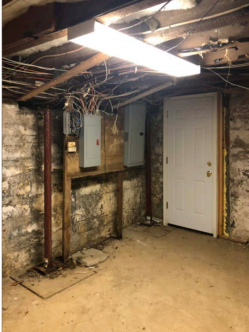
Photo 5. View to southeast within cellar, at the base of stairs within the bulkhead shown in prior photo. This area floods frequently. Current system of roof gutters, leaders & subsurface drains is both inadequate & corrupted.
