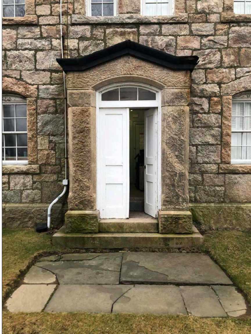
Photo 31. Tower (north) entrance and frontispiece. Aside from the errant electrical conduit to the left (east) and the cracked corner of the cast iron cornice, this entrance is in stunning condition. Bear in mind, too, that is has been the sole point of first contact for almost every major storm over the last 154 years.
