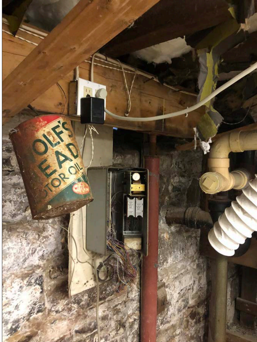
Photo 48. Myriad services and materials draped over, or attached directly to, the disengaged floor plate load transfer system.
