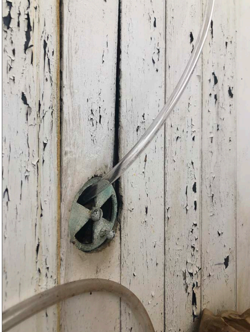
Photo 8. Detail of flexible tube routing rainwater collected from within the Lantern via funnels at the roof cove through the Lantern's original air vents (which, incidentally, were originally designed to regulate the lantern flame).
