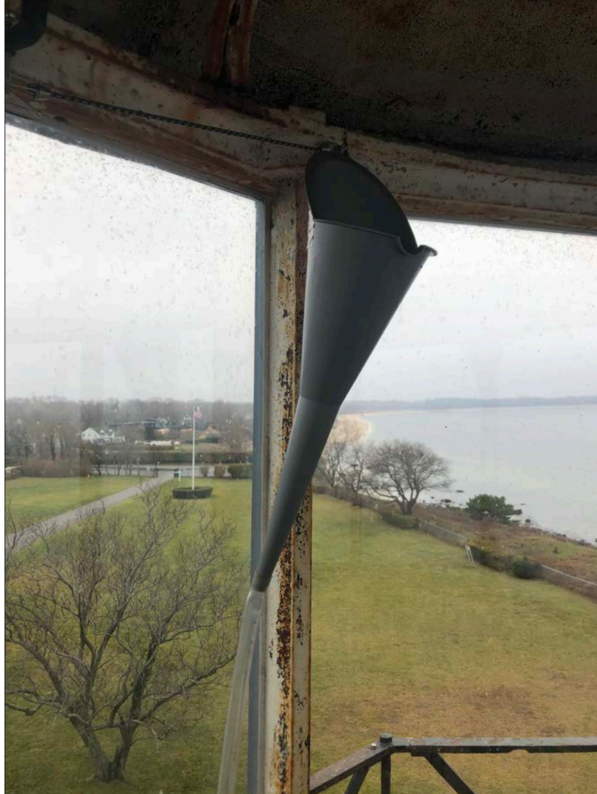
Photo 7. Detail of one of 6 funnels retrofitted to collect rainwater once it has penetrated the open joints of the Lantern roof.
