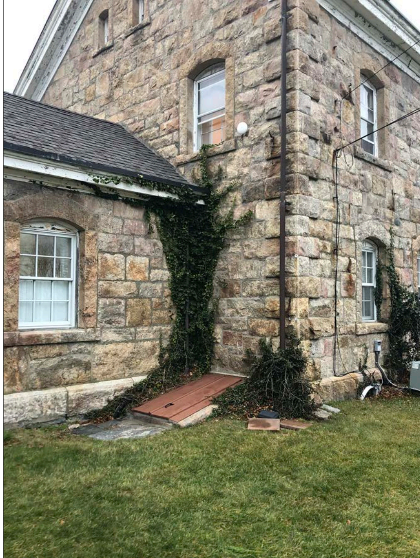
Photo 4. Stormwater collection and distribution systems are, generally, undersized and inadequately integrated. Subsurface drains are perhaps irredeemably clogged, resulting in water pooling at foundation, bulkhead stairs, and cellar door at base of bulkhead (adjacent to electrical panel). Rampant vegetative growth in southeast corner is supported by pooling water within the soil.
