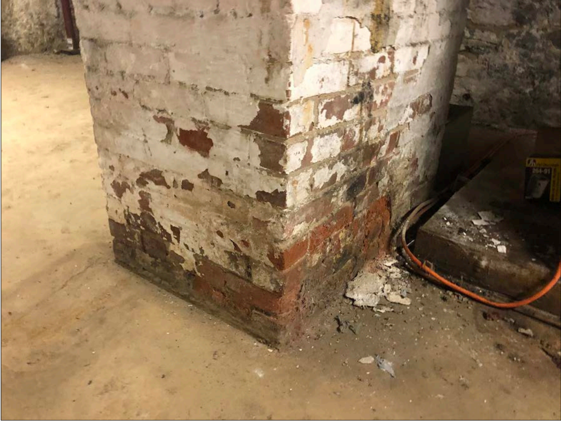
Photo 40. While common, pouring concrete floors over originally permeable cellar floors is extremely hazardous to the structural stability of porous masonry piers and foundation walls, because ambient groundwater that has always been present can no longer safely evaporate into the space (concrete is impermeable; it won't allow for moisture to transpire). Therefore moisture wicks up the only escape route available – porous brick masonry piers and foundation walls. The excess moisture and soluble salts forced into these structural systems begins a slow, measurable pace of structural deterioration. That is evidenced here by the spalling surfaces of the lower 4 courses, which will rise over time.
