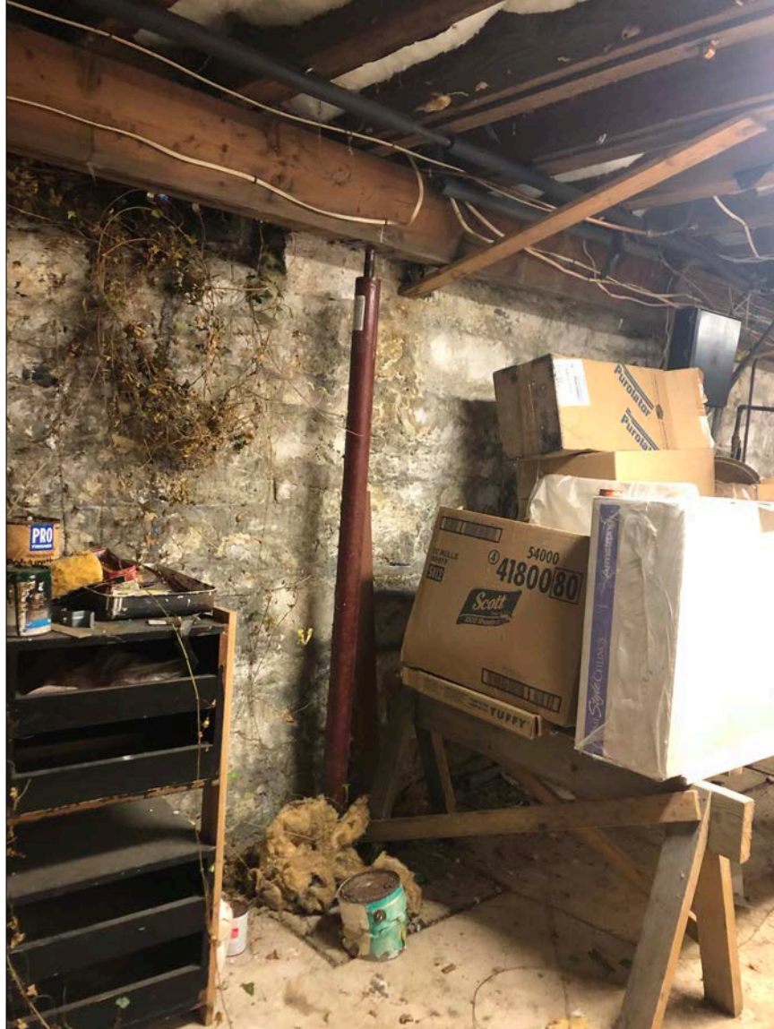
Photo 44. More of the cellar conditions described in Photo 43 above, along with accumulation of materials and debris. The square-formed concrete at the base of the column indicates that an independent pier is likely, which is positive, though the specifics of its design and installation are yet unknown.
