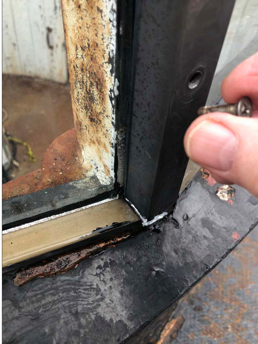
Photo 15. The original Lantern frame incorporates a superlative glazing bar system. Aluminum panning over the original glazing bars might have the appearance of an upgrade, but is corrosive to the underlying original system. It introduces a dissimilar metal (potentially producing a galvanic reaction), hides the condition of the original, relies only on weak sealants at corners, and is not secured to the underlying structure (the screw indicated – one of many – is just placed in the hole for show, not actually fastened to anything).
