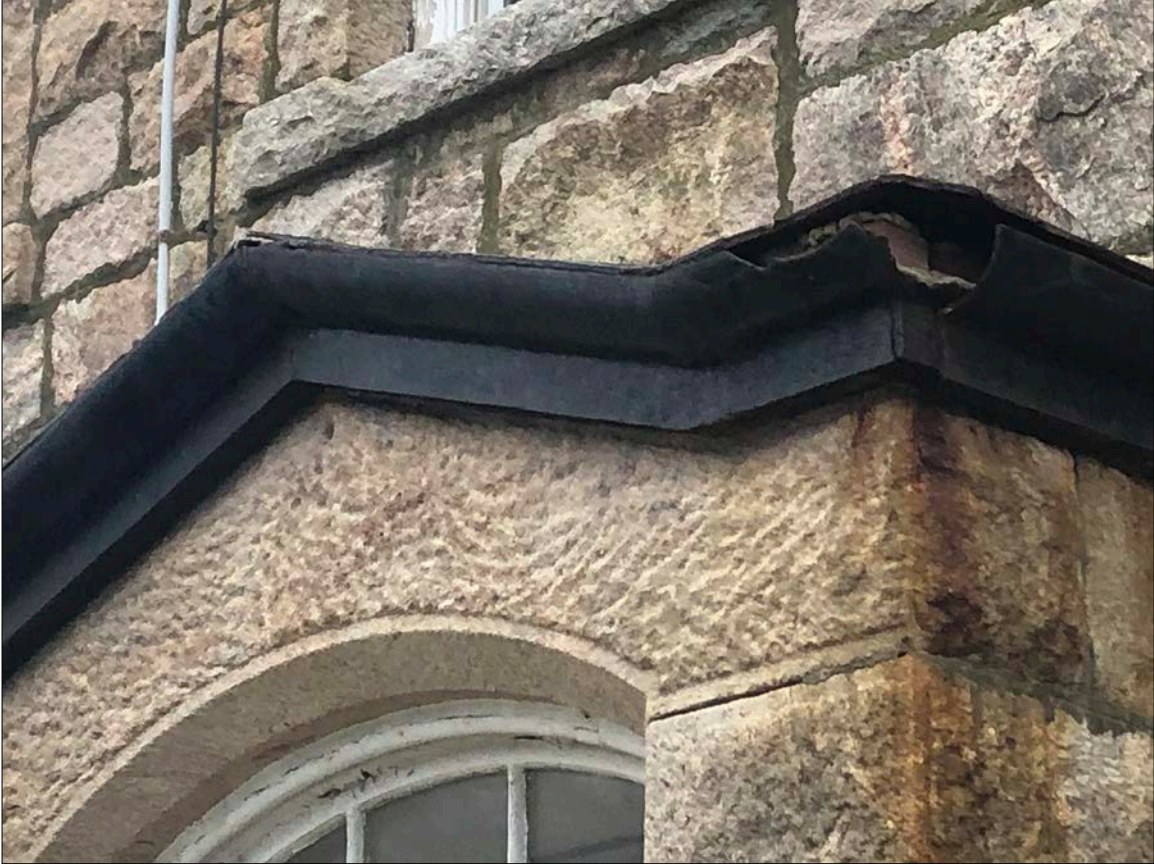
Photo 32. Detail of cracked corner of north entrance cast iron cornice. This is fully restorable, in cast iron (i.e., not alternative materials of lesser durability).
