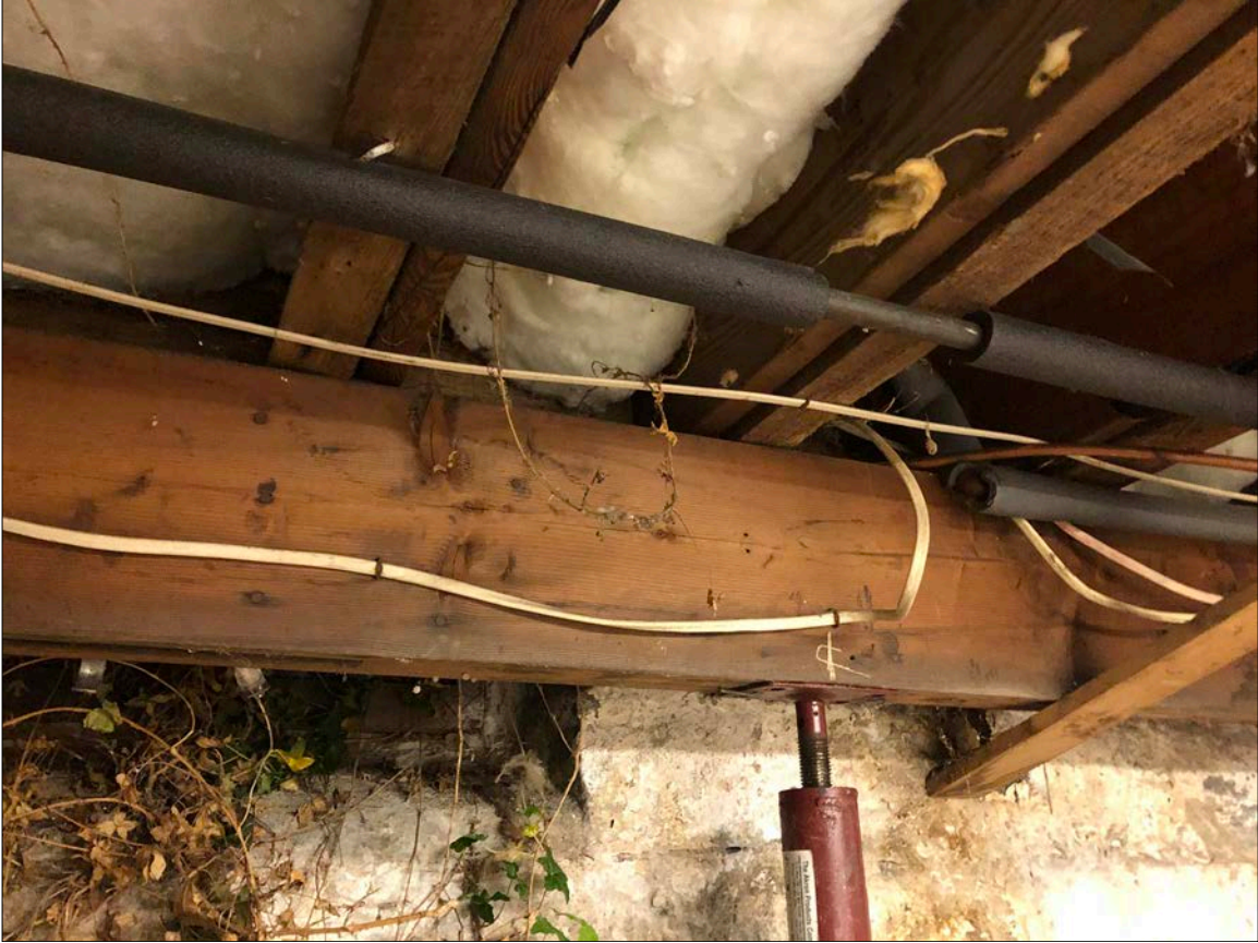
Photo 43. Many conditions of concern: 1) Disengaged floor plate; 2) Electrical wiring fastened to a girder that is inherently unstable (or, at least, structurally indeterminate); 3) Vegetation growing through the block ventilation window; 4) Blocked ventilation window(s); 5) Discontinuous insulation that is now partially trapping excess moisture within the cellar (rather than allowing it to dissipate naturally upward via convective heating, as the building's inherent design features intended); and 6) A confluence of issues so baffling that an untrained eye would find it difficult to discern where to begin... or why.
