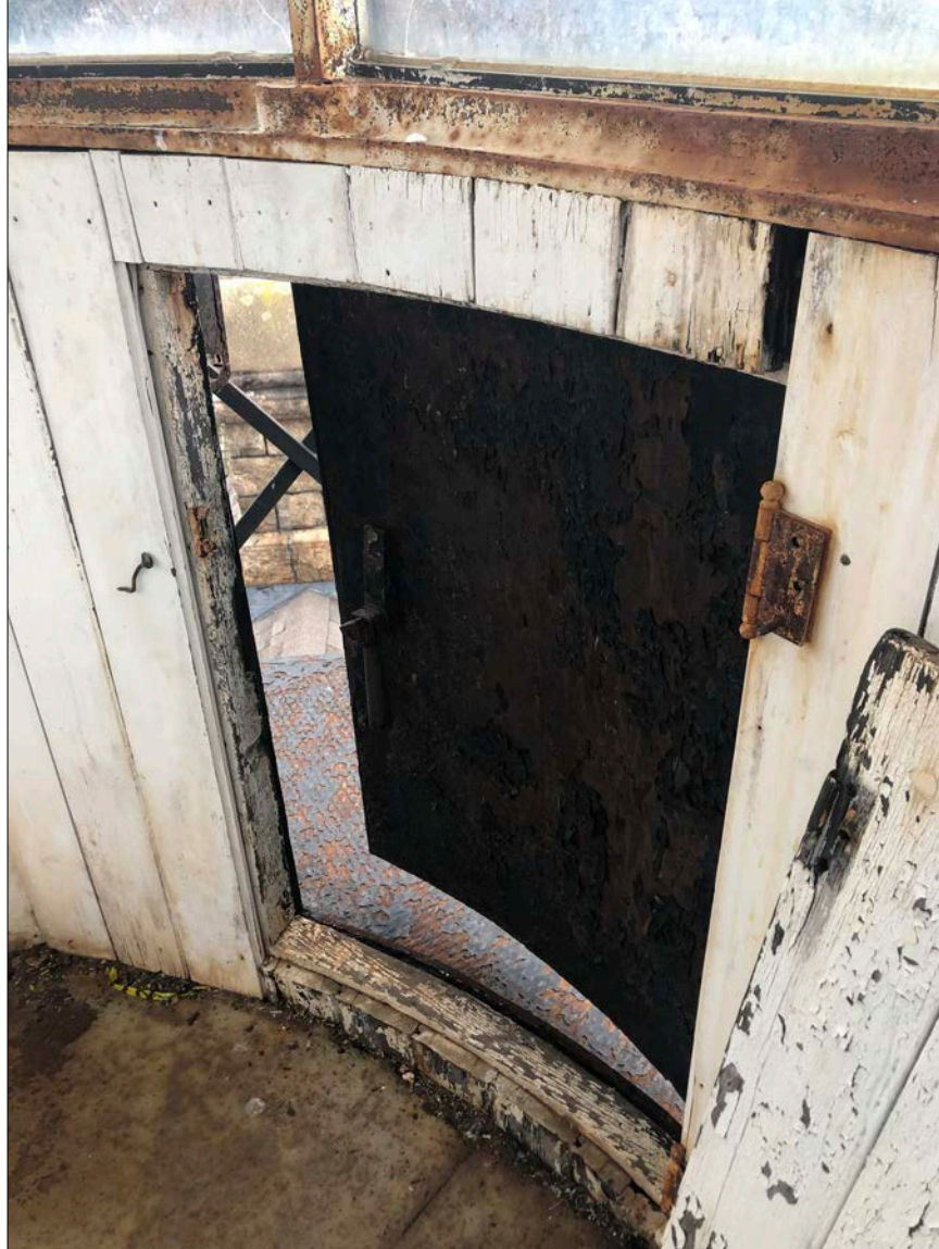
Photo 11. Lantern hatch to Lantern Gallery. This door is actually in sound working order fundamentally, although the application of inappropriate seals and deteriorating paint interferes with its smooth operation.
