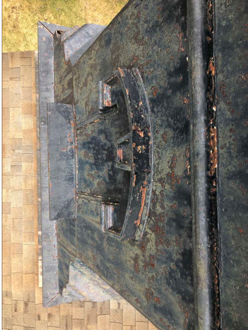
Photo 18. Looking down from Lantern Gallery, over railings. The condition of the Service Level facade plates, blind window hood & sill, and dated breastplate beneath them are in superlative condition. There are, however, significant breaches in the fascia directly under the Gallery, a particularly weak point for weathertight integrity, particularly when facing the direct brunt of salt laden storm water and high winds. All of it is readily restorable.
