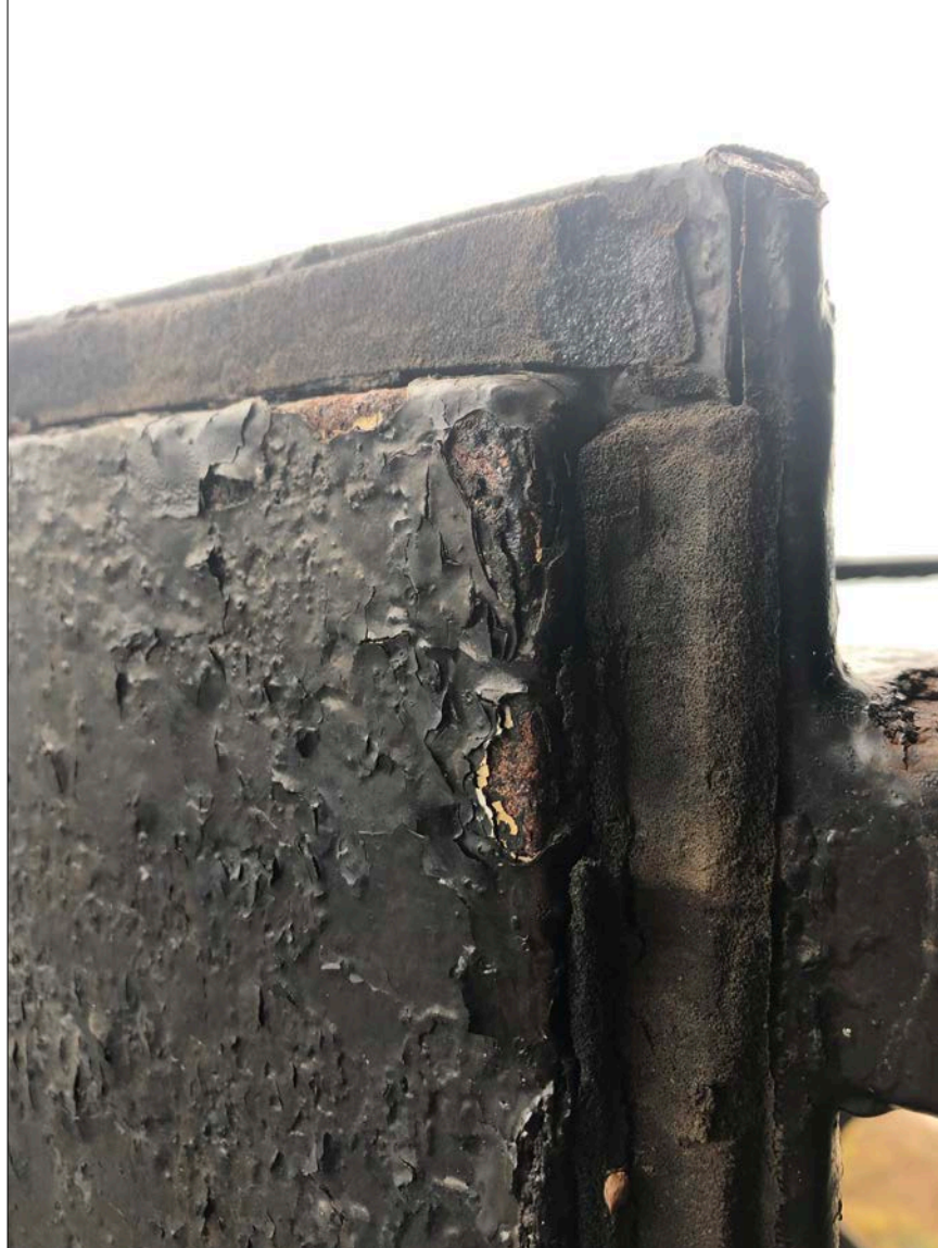
Photo 13. Detail of upper interior corner of cast iron hatch providing access from Lantern to Gallery. Note the addition of non-compressible perimeter seals as well as the build-up and deterioration of paint coatings.
