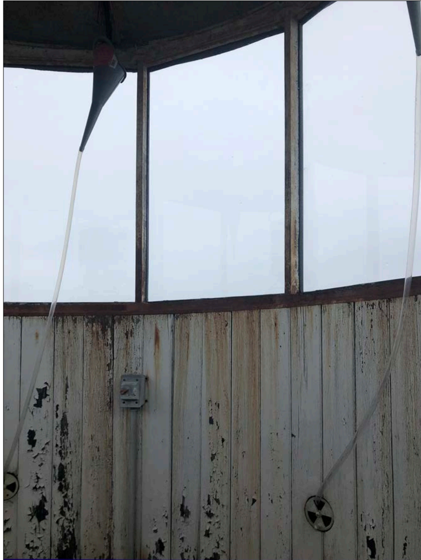
Photo 6. At the Lantern, an ad hoc system of funnels (6 total) collects rainwater from the interior of the cove, which is accessed via open joints of the ogee roof dome above. Water collected is channeled via clear tubing to the exterior deck of the Lantern Gallery, through the Lantern's air vents. This is neither a sustainable installation, nor effective: Properly repairing the roof and cove will keep rainwater out of the Lantern interior.
