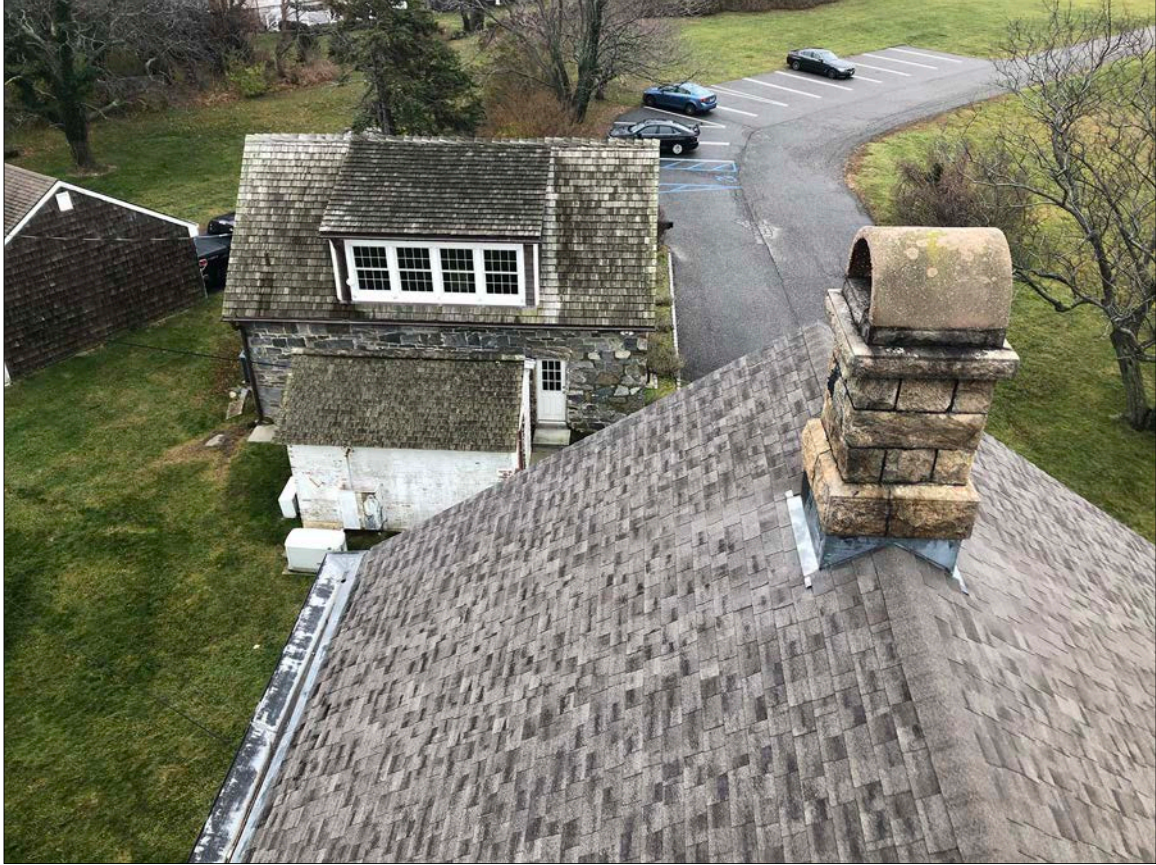
Photo 26. Composition shingle roof is nearing the end of its performance life. Chimney masonry and flashing remain in serviceable condition. Stormwater collection and distribution systems – gutters, leaders (downspouts) and subsurface stormwater conveyance components – are undersized, not well integrated, and clearly breached in numerous critical locations. The condition of subsurface elements is, on the whole, a complete mystery; further investigation, via a drain scope, is warranted.
