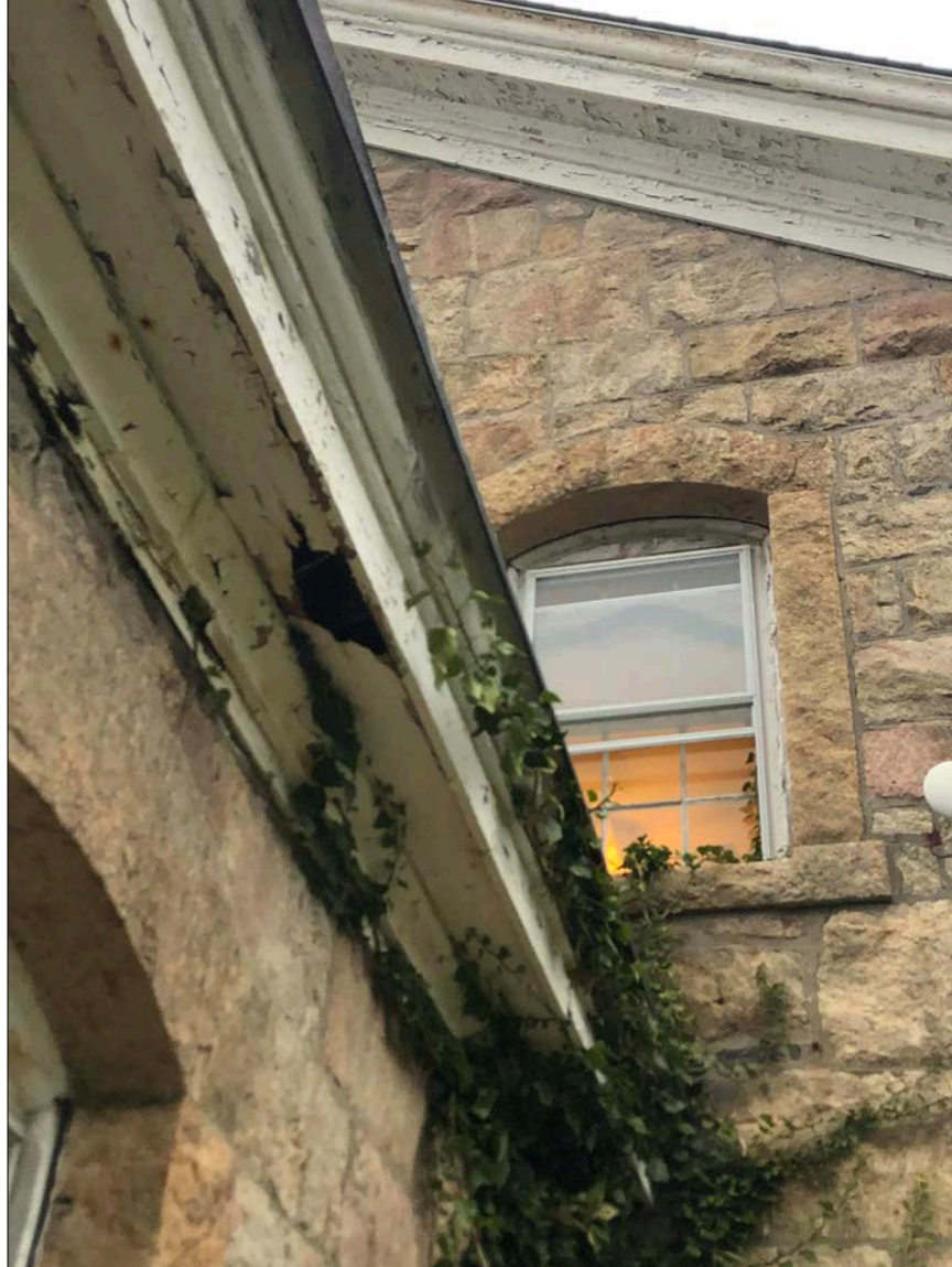
Photo 36. Breaches in the stormwater collection and distribution system have led to serious degradation of structural framing and soffits, and have fed rampant vegetative growth occurring in the building's southeast corner.
