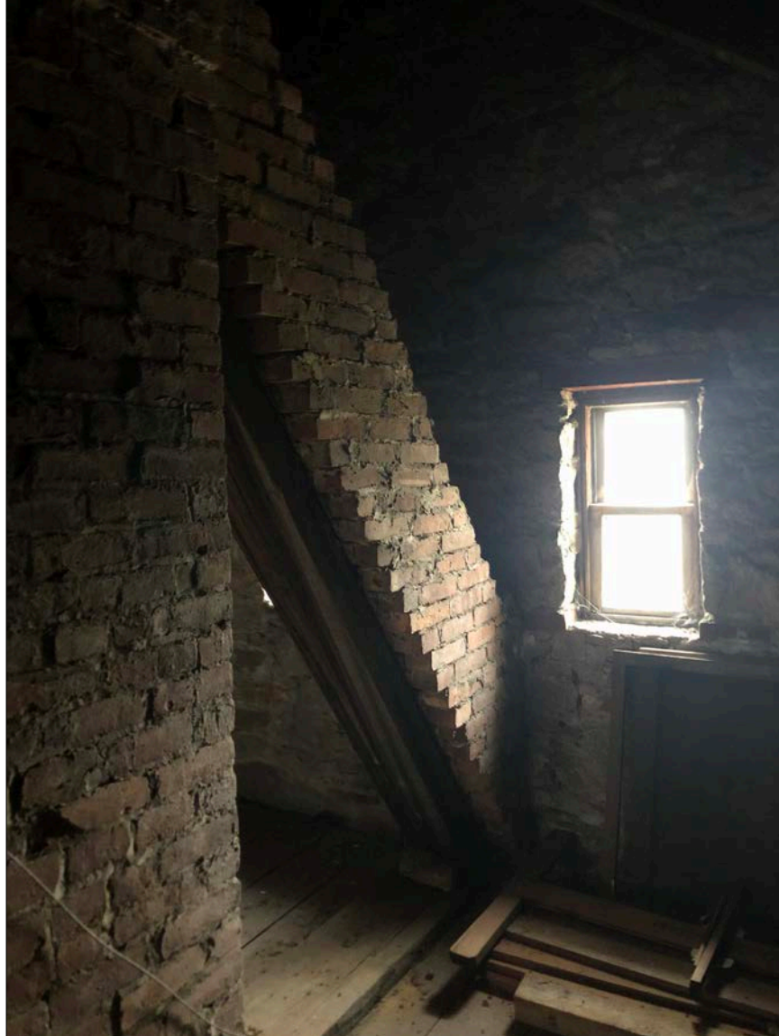
Photo 45. A corbelled flying buttress providing lateral support of the original brick chimney is engaged and in stable condition; this is an original element.
