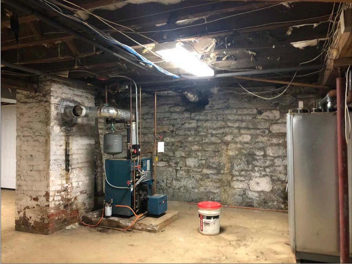
Photo 46. A relatively new boiler, skillfully piped, serves as the heart of the Lighthouse's oil-fired closed-loop hydronic heating system, which is distributed within habitable space via cast iron radiators, most original. This is an exceptionally efficient system for a building of solid masonry construction.
