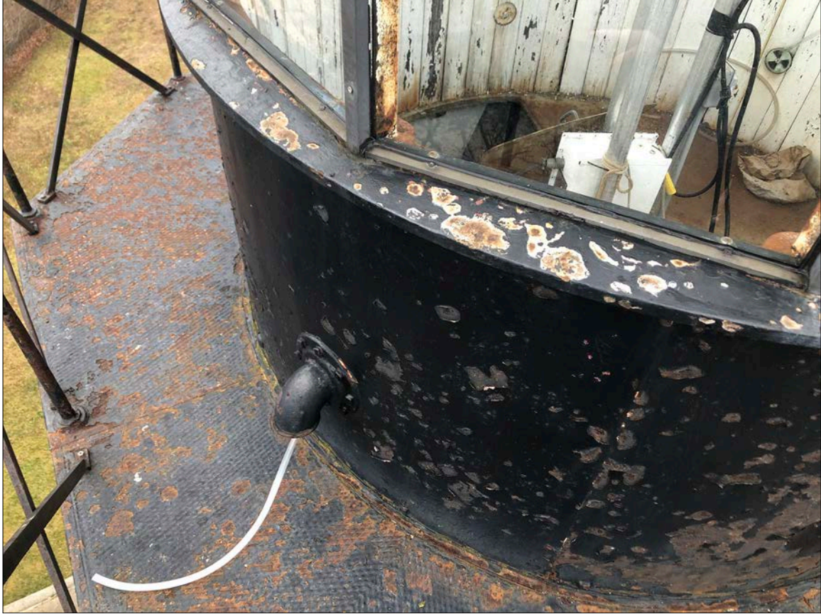
Photo 17. Lantern Gallery embossed decking, original circular drum and sill, modified railings. Note flexible tube from funnel collection system protruding through original air vent terminus.
