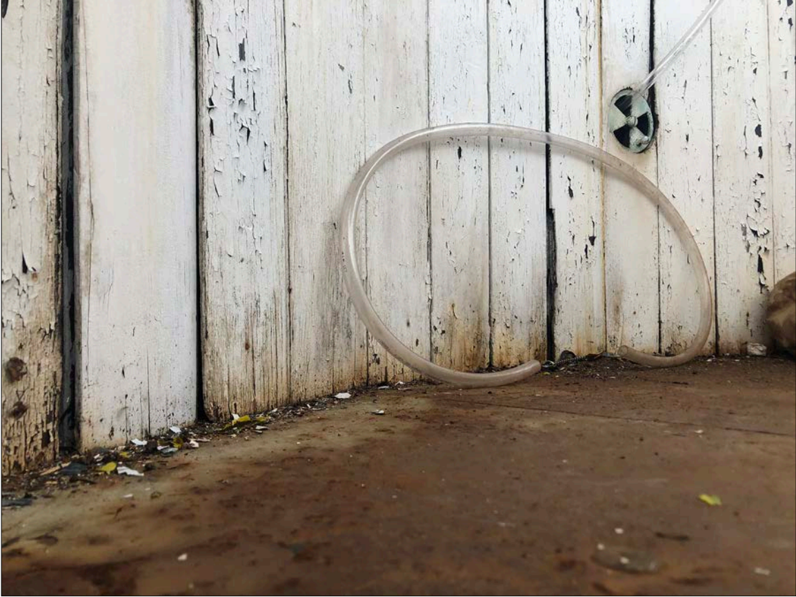
Photo 20. Interior Lantern drum vertical tongue-and-groove paneling. The end grain of wood readily absorbs water/moisture, and is where pathologies of deterioration often begin. Note the damage to paint associated with end grain at the base of the paneling.
