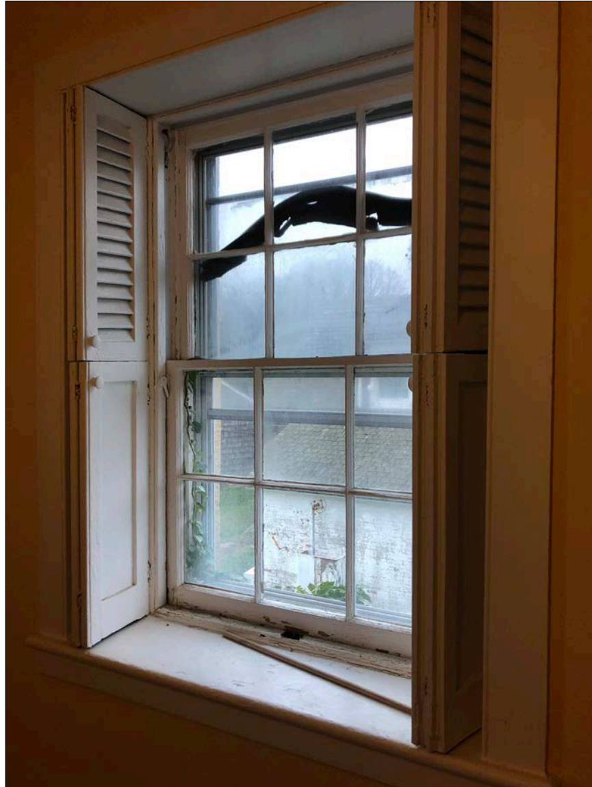
Photo 28. Early double-hung wood windows are in remarkably excellent condition, despite being somewhat sealed in by exterior triple-track storm windows. Note failing (dislodged) dry seals within the interstitial spaces, as well as encroaching vegetation and a stuck-in-place outer sash. There are far more effective ways to treat the windows and ensure superior energy, ventilation and visual performance. The integral blind shutters are beautiful.
