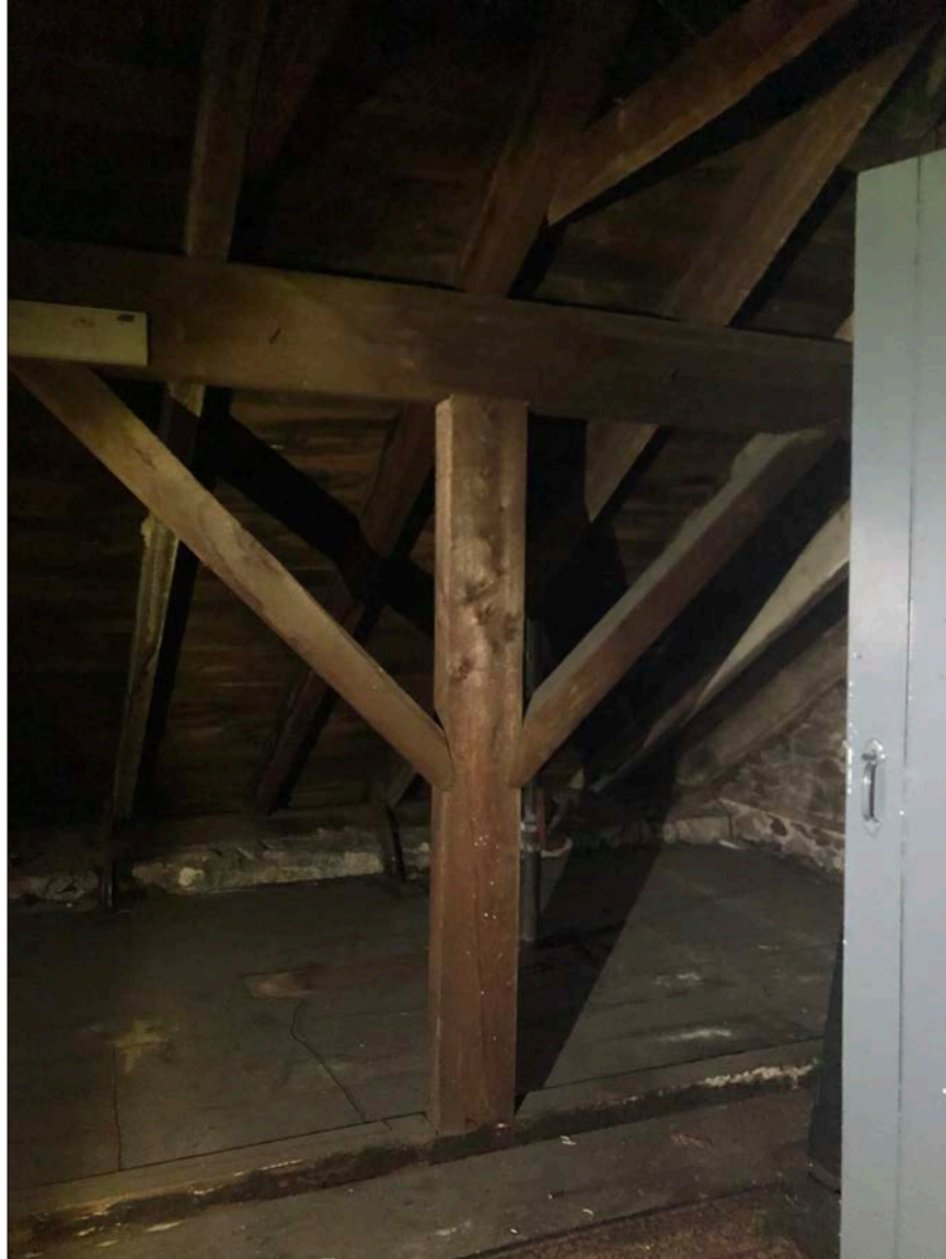
Photo 39. In contrast to the previous two images, for areas located away from the eave gutters, original framing remains robust and pristine.
