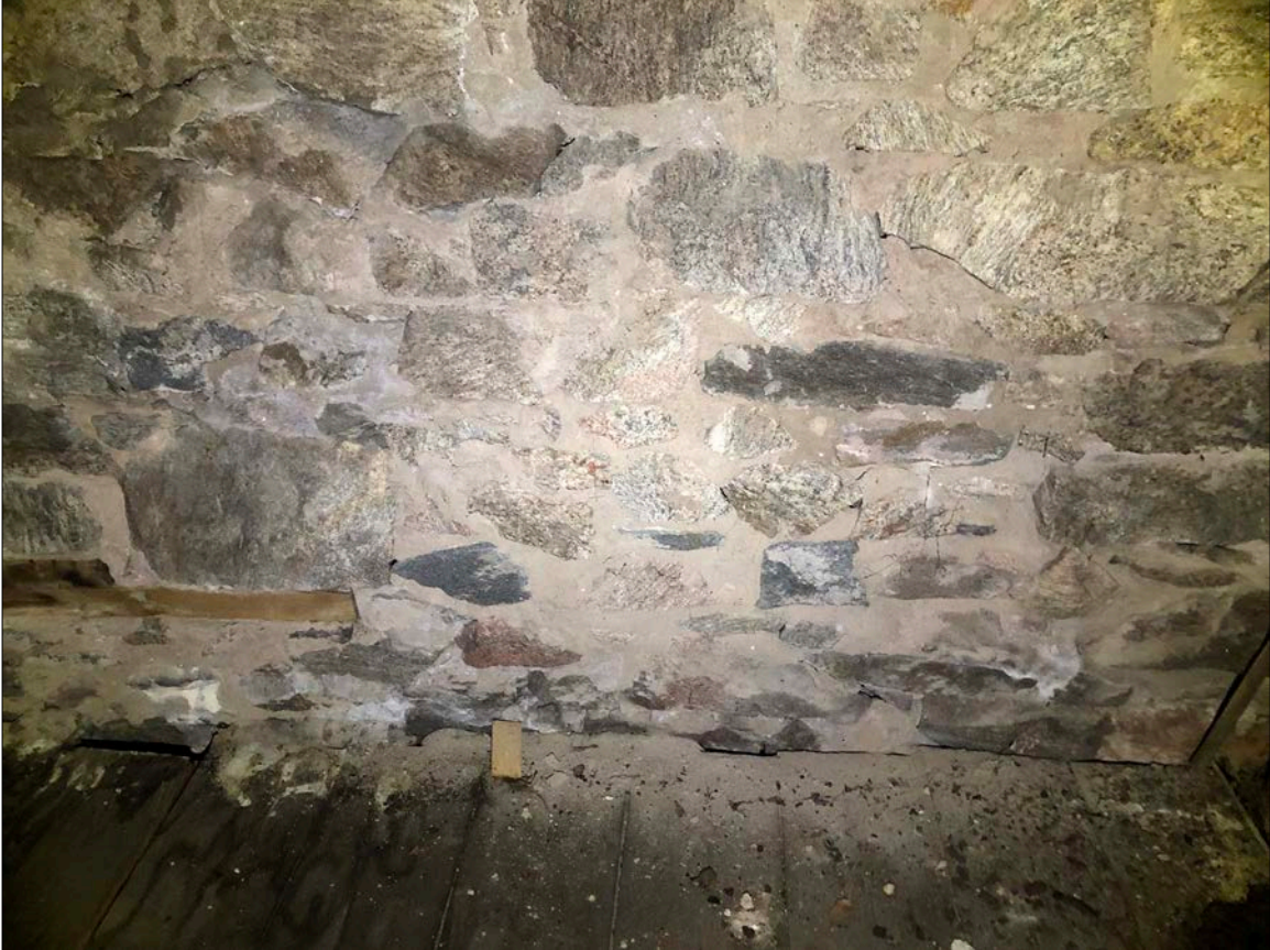
Photo 27. Upper wall system seen from the attic in the vicinity of the roof eave, where leaking gutters have led to water migration through the stone. Dusting on the adjacent attic flooring is indicative of microscopic degradation of mortar matrix. While not of particular concern, it is worth monitoring.
