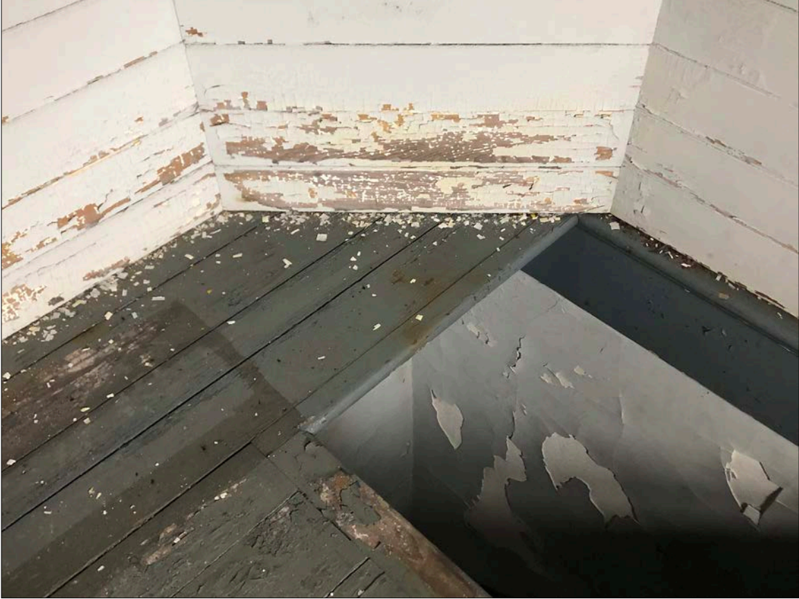
Photo 21. Horizontal tongue-and-groove paneling of the Service Level, which is bound by cast iron facade plates. Paint loss is indicative of moisture collecting behind the paneling; water likely accesses this location from the vicinity of the Watch Deck level above.
